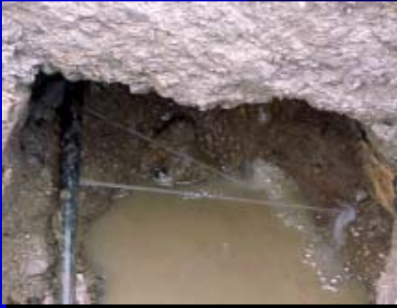
Water leak at Reynosa
